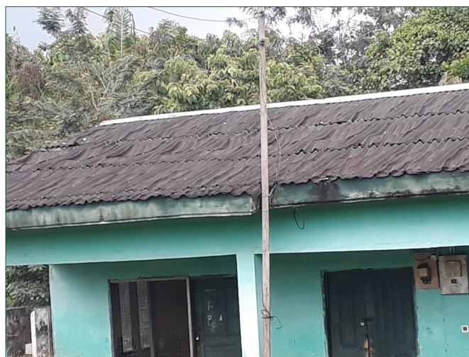
School roof repairs needed
